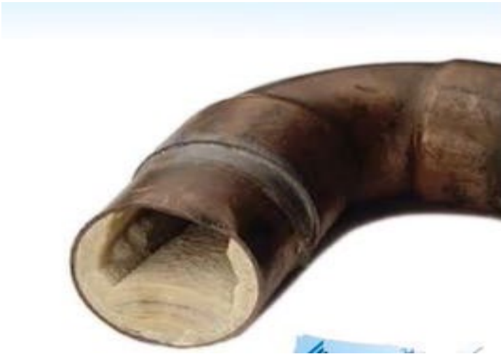
Calcium carbonate scale on a piece of pipe.
