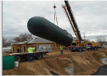
In-ground Storage Tank
